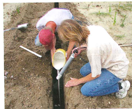
Contact water was captured through use of 10 ceramic collection suction tubes known as lysimeters placed underneath and surrounding the active composting pile (lysimeter installation shown in photo).
